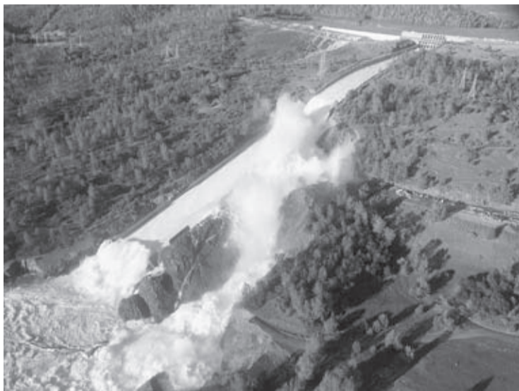
This Feb. 11, 2017, file aerial photo released by the California Department of Water Resources shows the damaged spillway with eroded hillside in Oroville, Calif.
